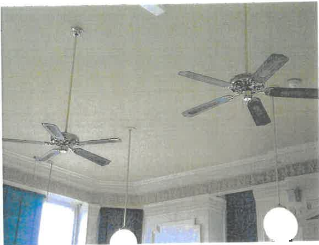
Figure 8: Ceiling fans in main restaurant space
