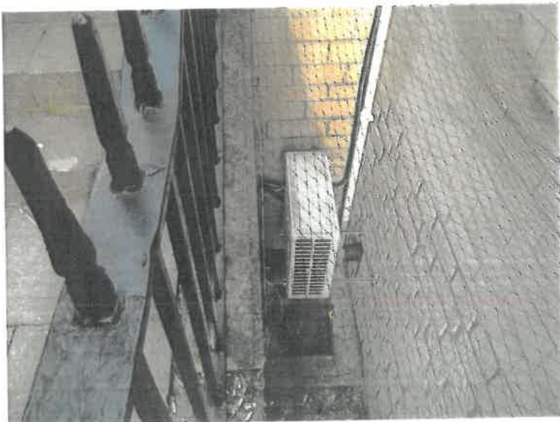
Figure 9: Outdoor unit on west side of building
